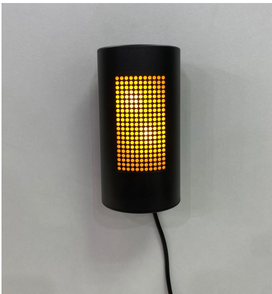
Figure 5: Example of CO 2 stoplicht attached to the wall by wall bracket.
